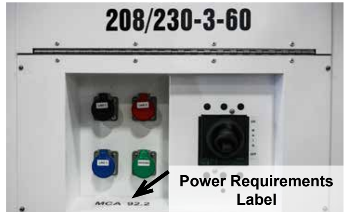
Figure 4 – Camlock Power Connections
