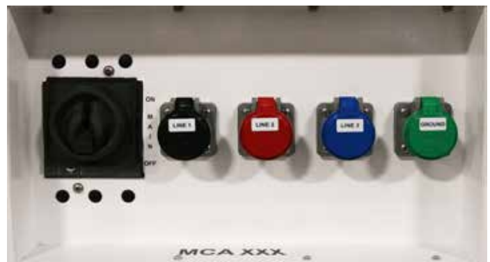
Figure 4 – Camlock & Circuit Breaker
